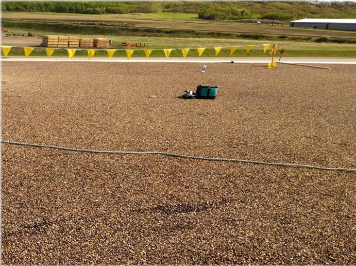
Worn out Tar and Gravel with Asphalt Emulsion ready to be installed
