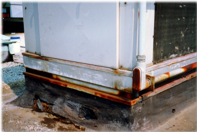
This asphalt BUR curb suffered from many years of UV degradation
