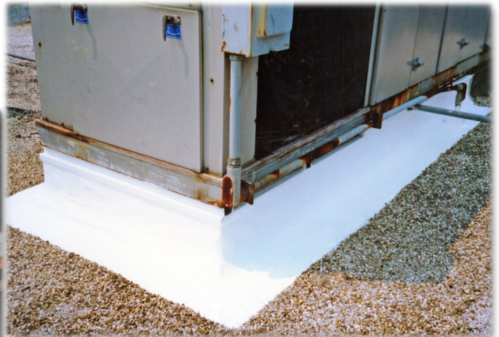
The Acrylabs Patch Kit was the perfect tool for making the repair and creating a watertight curb
