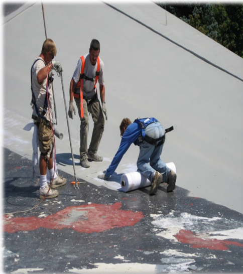
An excellent example of how the Acrylabs Fabric Reinforcement contours to the unique shapes of this roof
