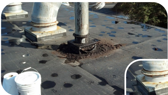
Heat destroyed EPDM Roof
