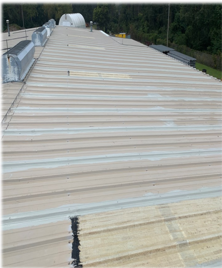
Fiberglass skylights are hard to see and create a dangerous hazard on roofs
