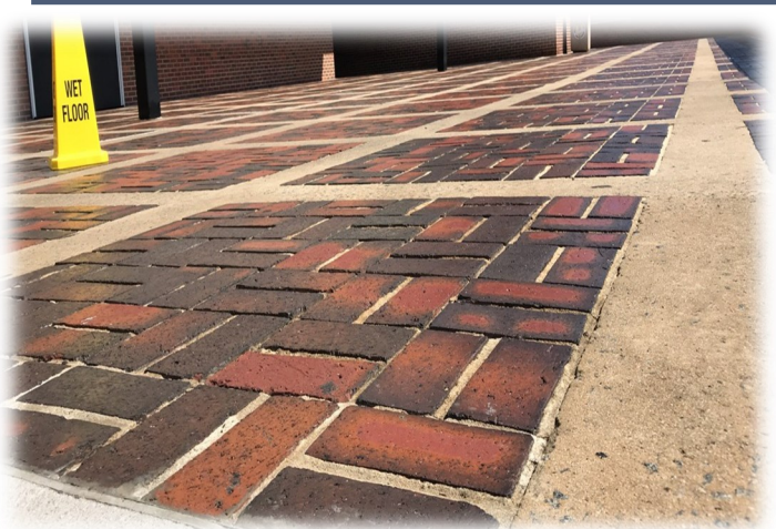
Brick, mortar and concrete were all treated with Acrypel to stop water intrusion and to protect the attractive plaza at a university campus
