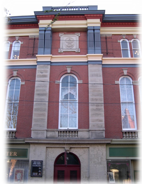
The exterior restoration of an historic Masonic Temple began with removal of old coatings to expose the original brick and masonry and Acrypel was then applied as a water repellent to preserve the surface
