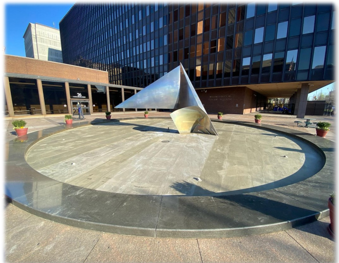
This center-city fountain is the pride of the block. Installing the Acrycrete System restored its vibrant look and provided a watertight surface
