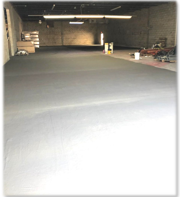
Damaged manufacturing and warehouse floors are expensive to replace. Acrycrete can solve a variety of floor issues with minimal disruptions of operations
