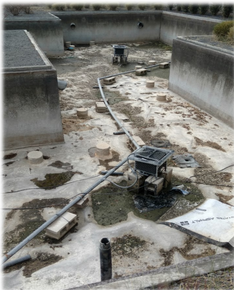
Drained lagoon exposing failures
